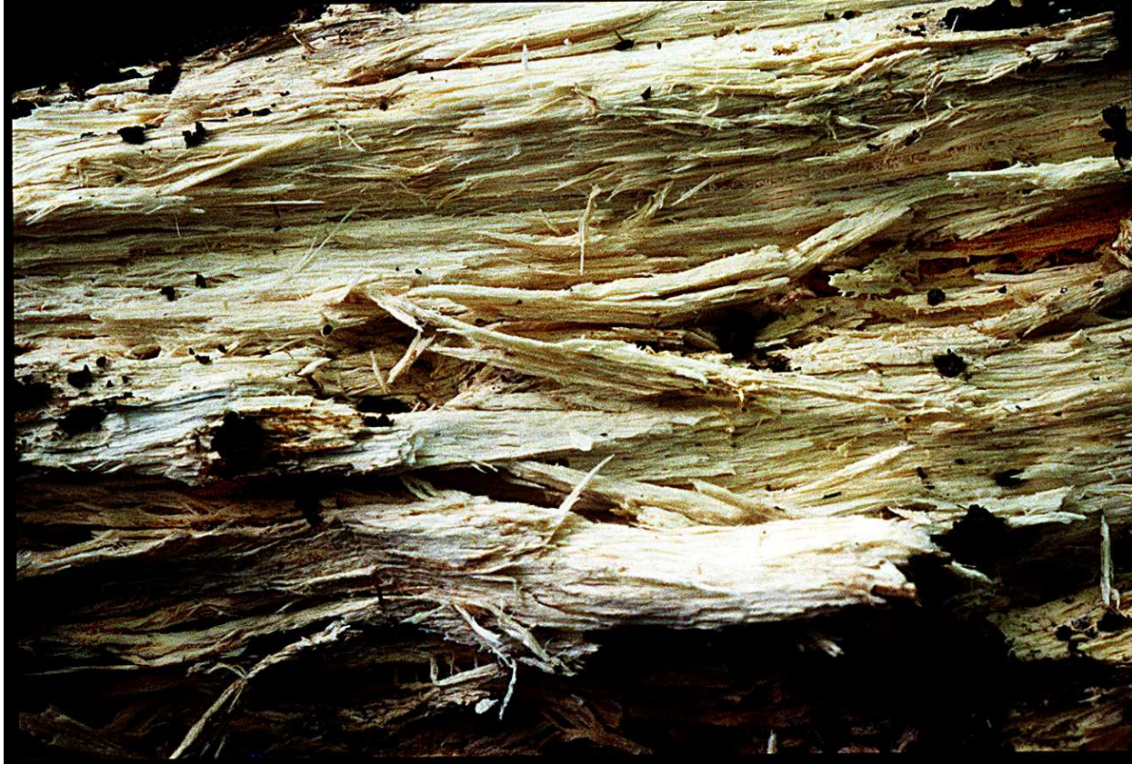
White rot: Cellulose and lignin decayed, stringy or spongy
