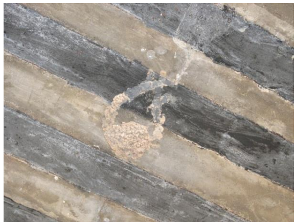
Figure 7-27: Potential swallow nest under a bridge.
