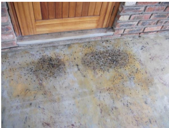
Figure 7-1: Bat droppings from bats roosting under roof of building.
