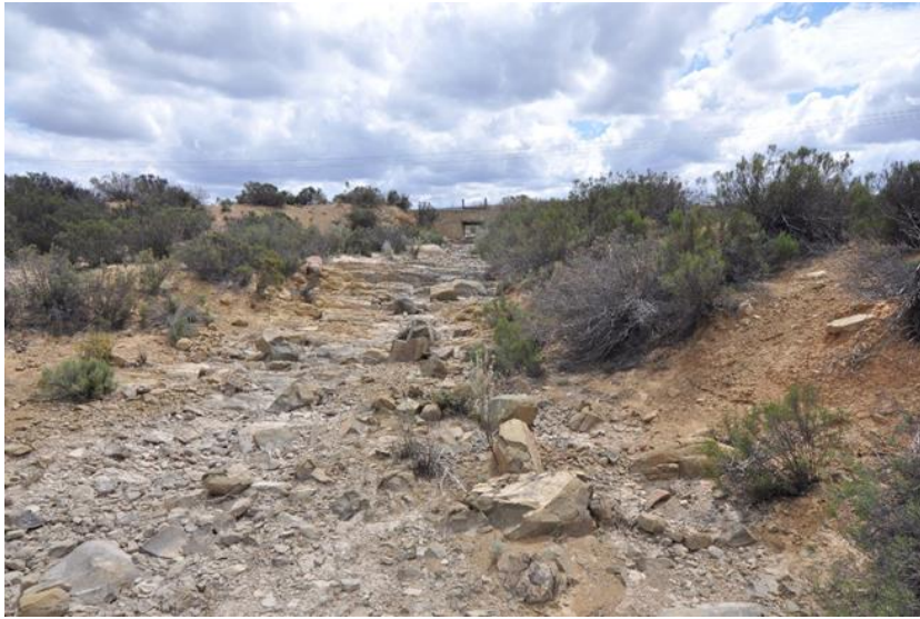
Plate 1: River bed erosion below an existing culvert.
