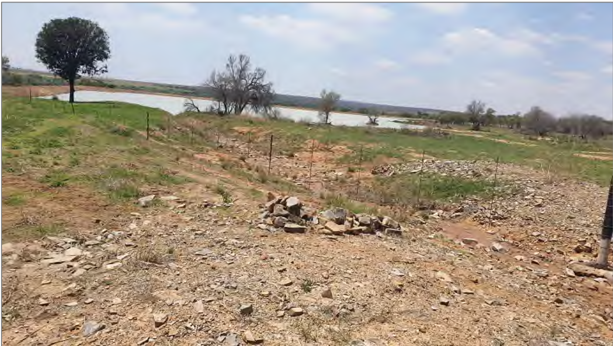
Figure 11-5 Instream impoundment and soil disturbance (Taken October 2020; 24°12'53.07"S; 27°57'38.25"E)
