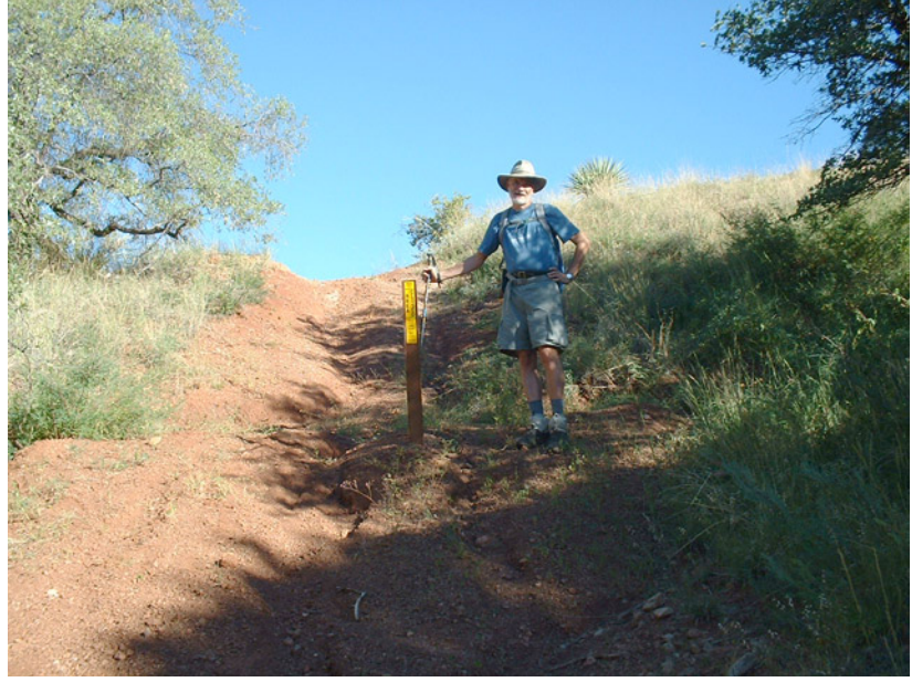
Figure 5.3 Erosion from a poorly-conceived road.
