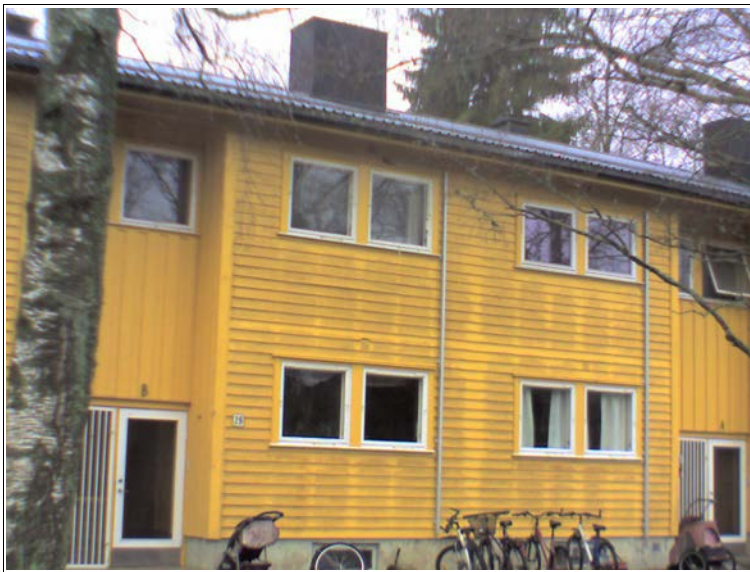
Figure 6. Mould growth on coated wooden cladding on a residence house in Ås. Photo: Precision Technic Nordic.
