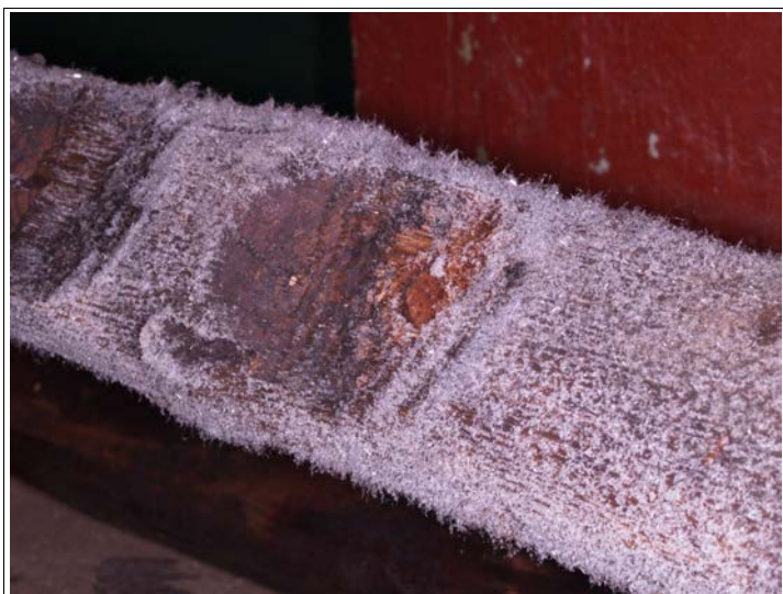
Figure 4. Accumulated salt crystals on wooden surfaces in a crawlspace under buildings at Bryggen in Bergen. Photo: Mycoteam as.
