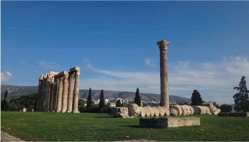
5.16 A collapsed column showing typical drums of which the column was made.
