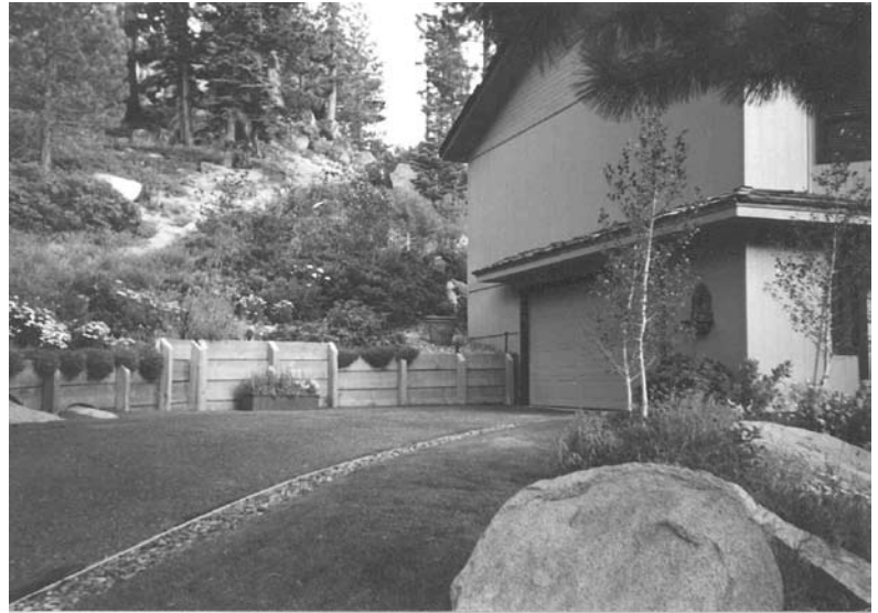
Sven Krevold and Dan Sutton won TRPA's Landscape Design Award for this slope stabilization, revegetation and driveway paving project. (See close-up, Page 24.)
