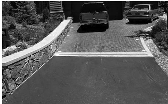
Above, driveway runoff is directed to a slotted channel drain, which conveys water to an appropriately sized system for storage and infiltration. Note the rock borders along the driveway, which can infiltrate water and prevent soil and nutrients from moving onto the paved surface.
