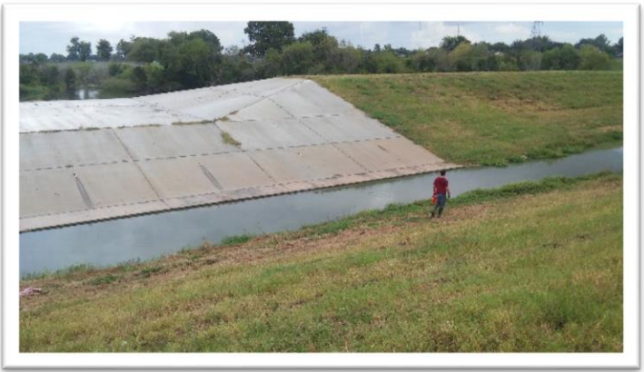
View of the site from the top of the adjacent slope, October 2016
