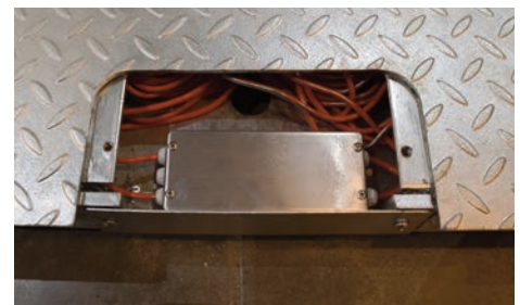
Internal view junction box Galvanized base
