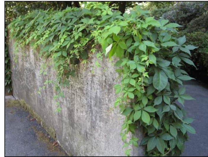
Figure 4.3.17-2 Concrete Wall with Vegetation
