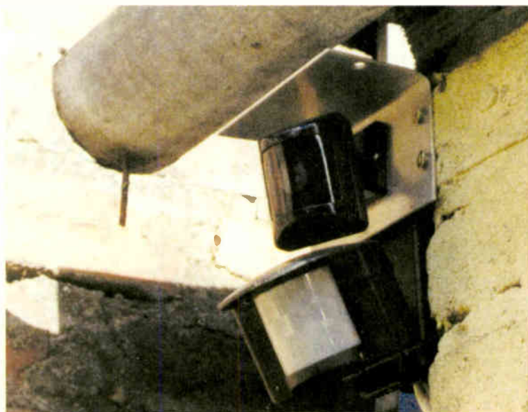
Sensor using the PIR housing from a defunct security lamp.
