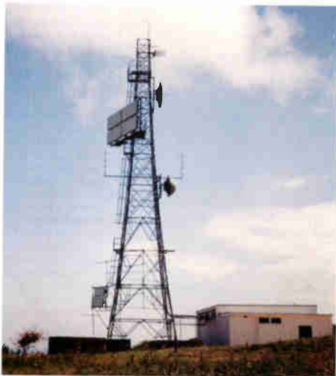
The Alderney TV relay transmitter and mast. Sabre is the large boxed panel near the top of the lattice structure. The local group C/D transmission aerial is the thin vertical element atop the mast.
