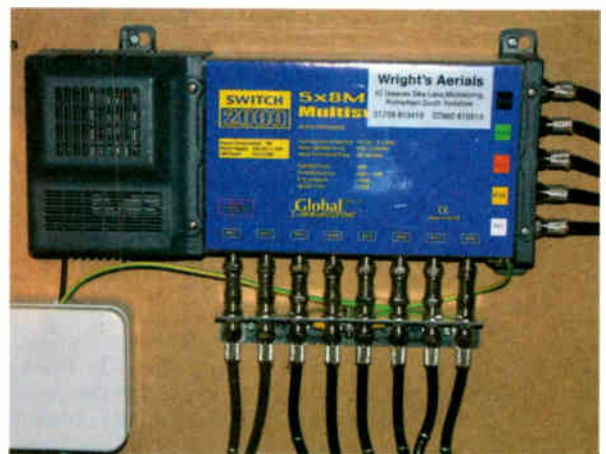
Figure 3: A Global 5X8M mains-powered multiswitch in place. The one terrestrial and four satellite inputs are on the right, with the outputs along the bottom. This photograph was taken before the installation was earth bonded.
