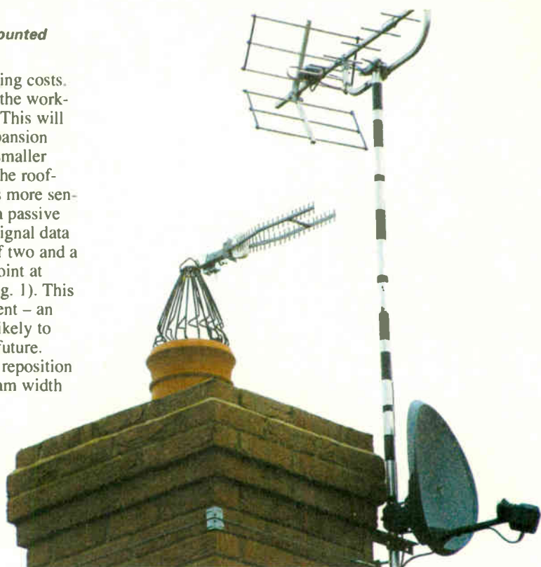
An external broadband data-link aerial for domestic use.
