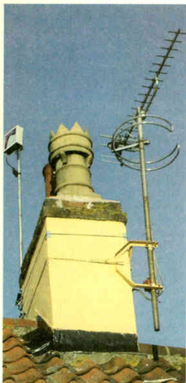
Left: Steve's chimney-mounted data link.
