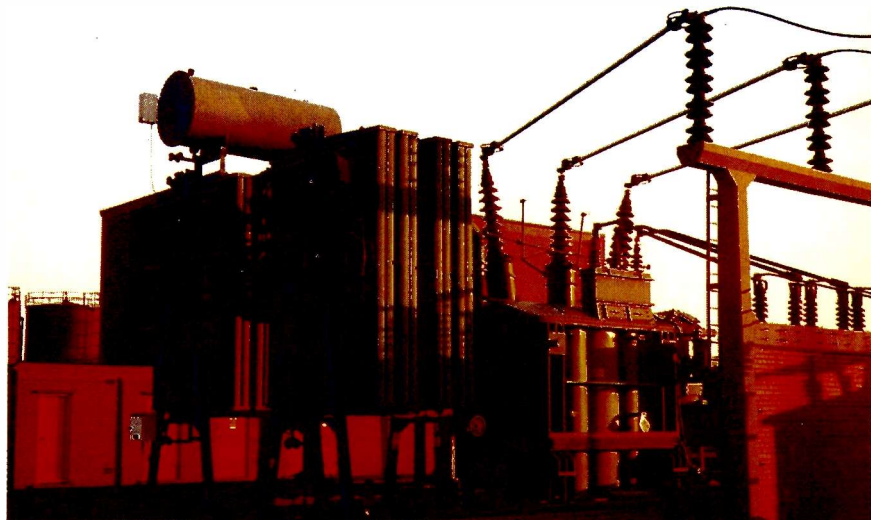
A 132kV substation transformer with forced cooling.
