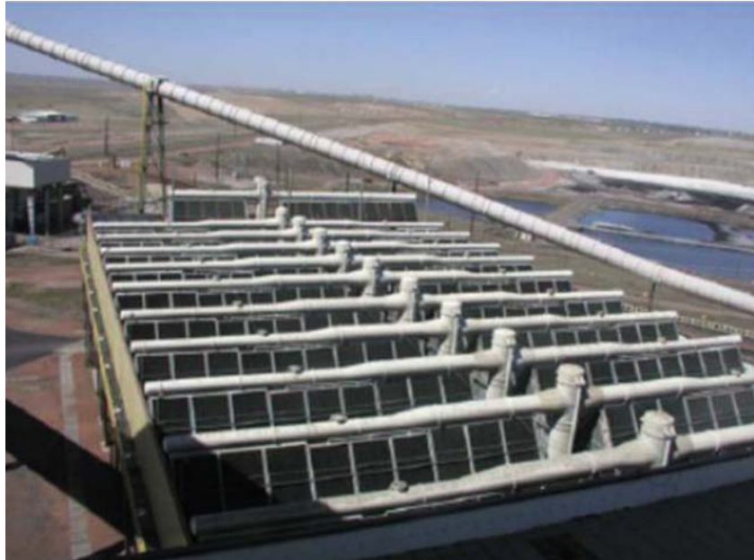
FIG. 40. Actual picture of air cooled condenser with forced draft fan units at Pacific Corp Wyodak power plant, Gillette, Wyoming (Courtesy EPRI).
