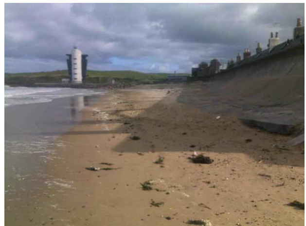
Figure 8: Exposed seawall foundations at Footdee, Aberdeen, UK. Summer, 2010 (Guillaume de la Fons)
