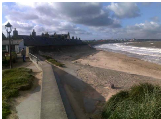
Figure 9: Damaged seawall at Footdee, Aberdeen, UK. Summer, 2010 (Guillaume de la Fons)
