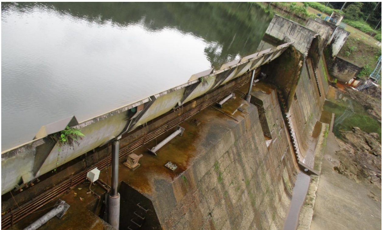
Above: the three Kingulé power lines (3 x 20 m 3 / s), below, Kingulé dam Kinguélé plant and dam (SEEG)
