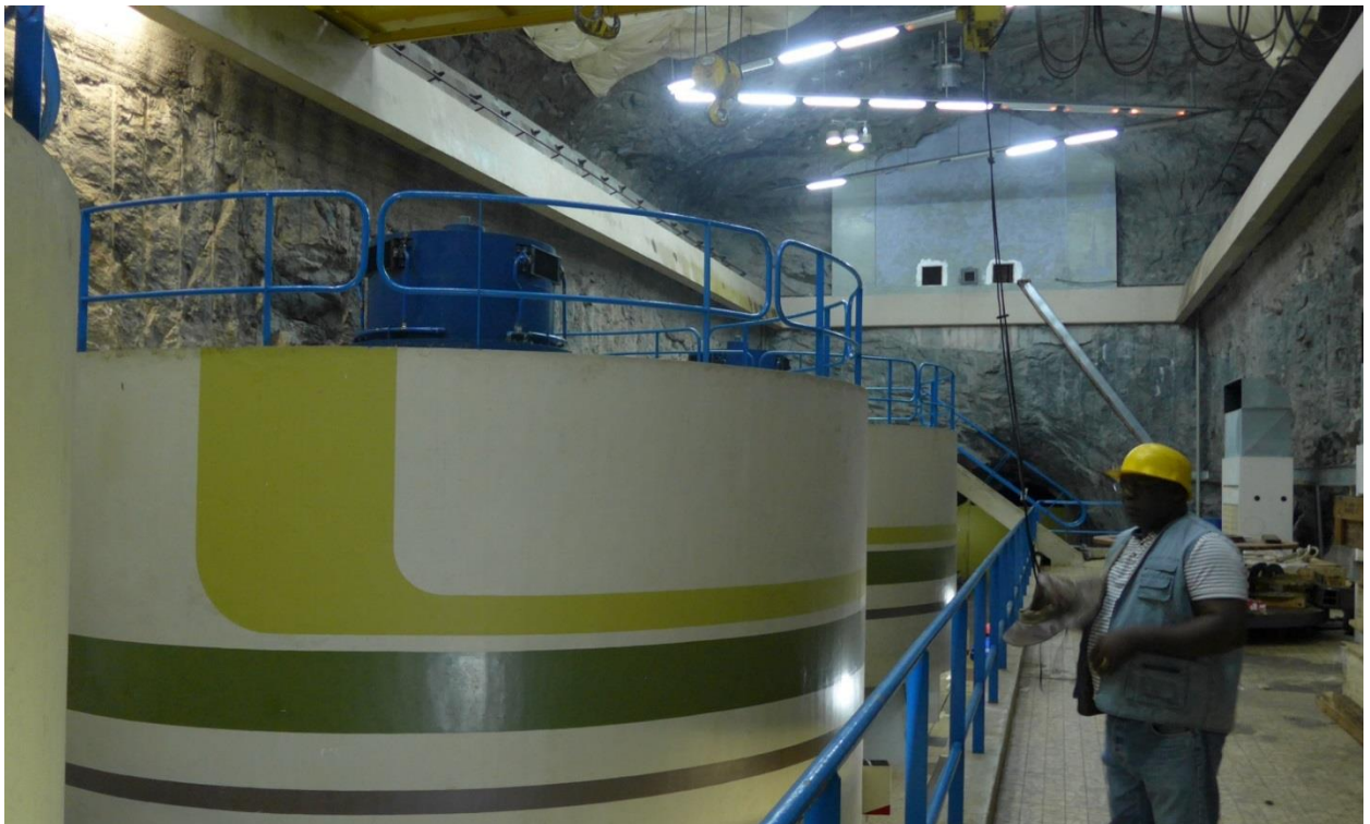
Lake and Tchimbélé powerhouse (SEEG)
