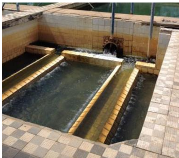
Figure 1. Image of one of the filters during the backwash process.
