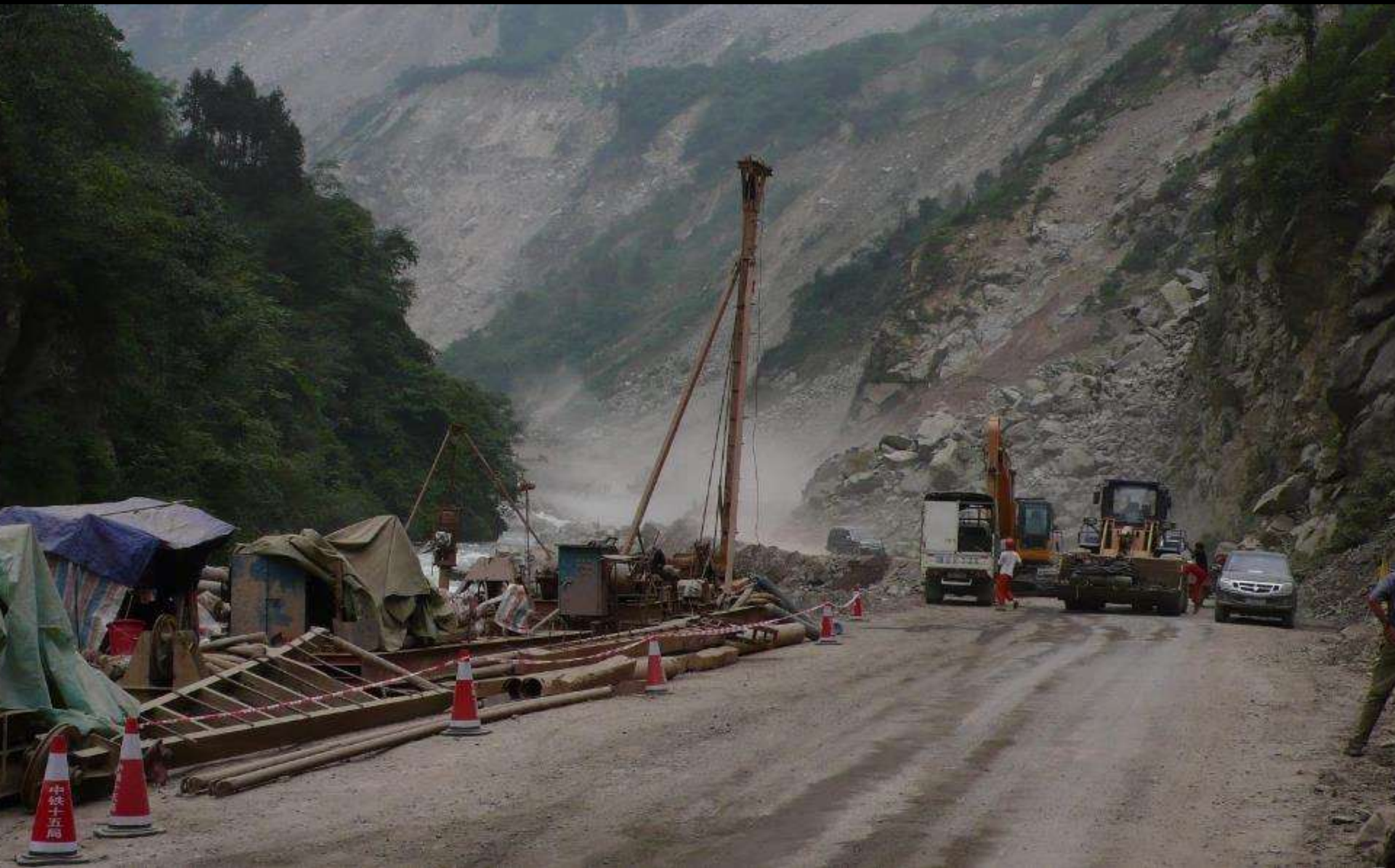
Road through the Wolong Nature reserve after the tragic Great Wenchuan earth quake of 2008
