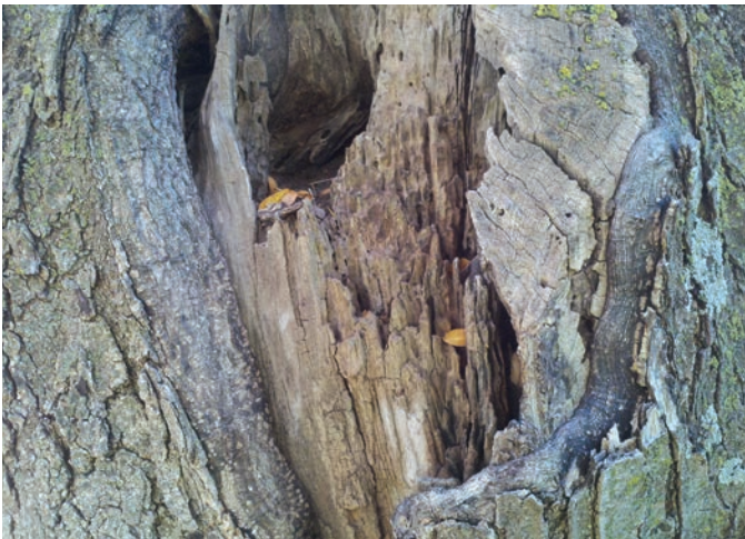
Photo 39. Crumbling wood indicates decay.
