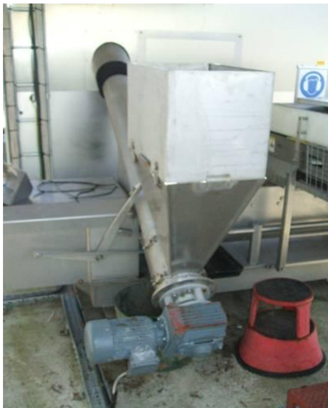
Figure 9: Hopper installed over the 'in-auger' to help adding co-feedstocks to macerated food waste.
