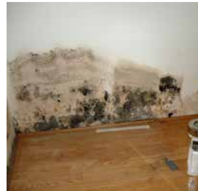
Air sampling taking place in a property where a leaking shower has caused extensive fungal growth (photo: G. Godwin-Keene)
