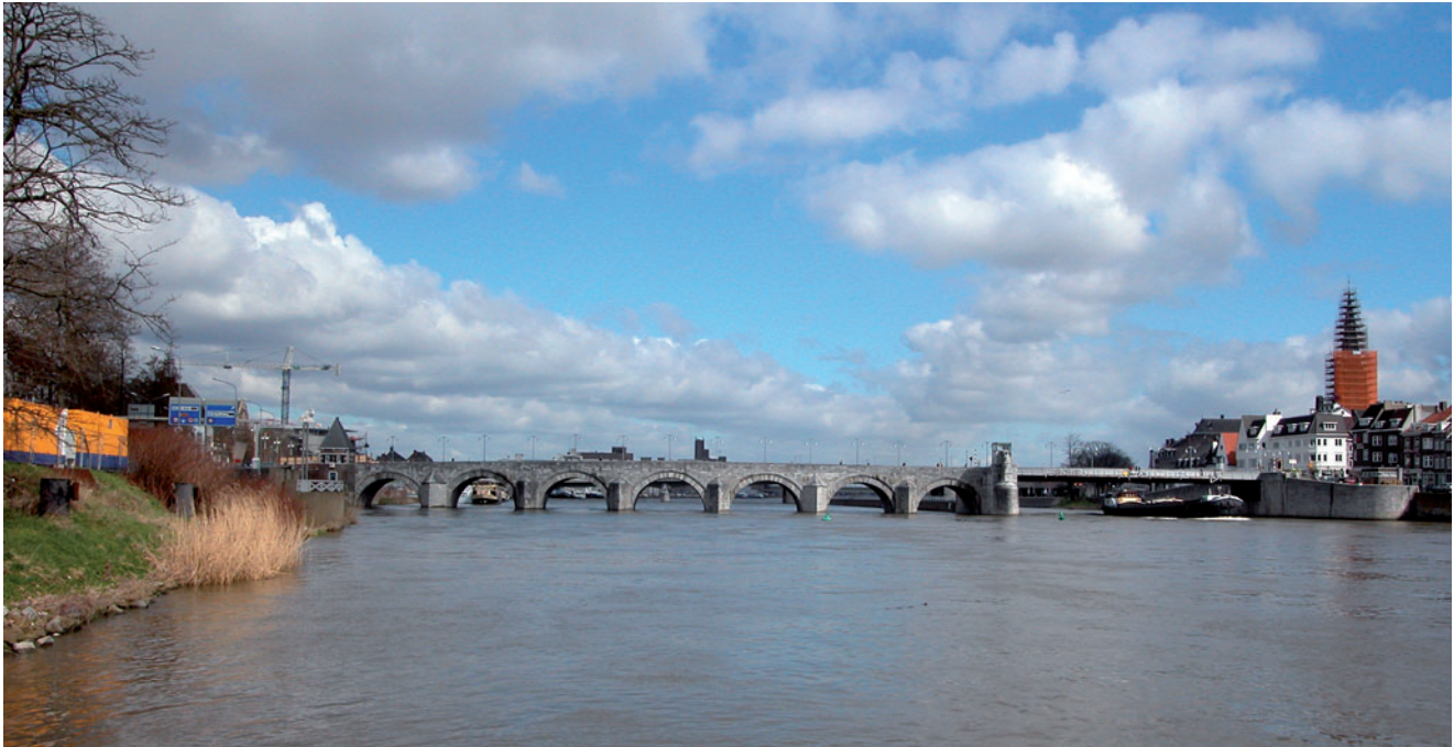
Fig. 14. St Servaas bridge, restored pillars are made of Bathonian limestone from France.
