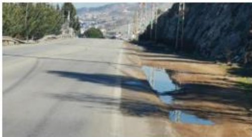
Drainage problem and damaged guardrails
