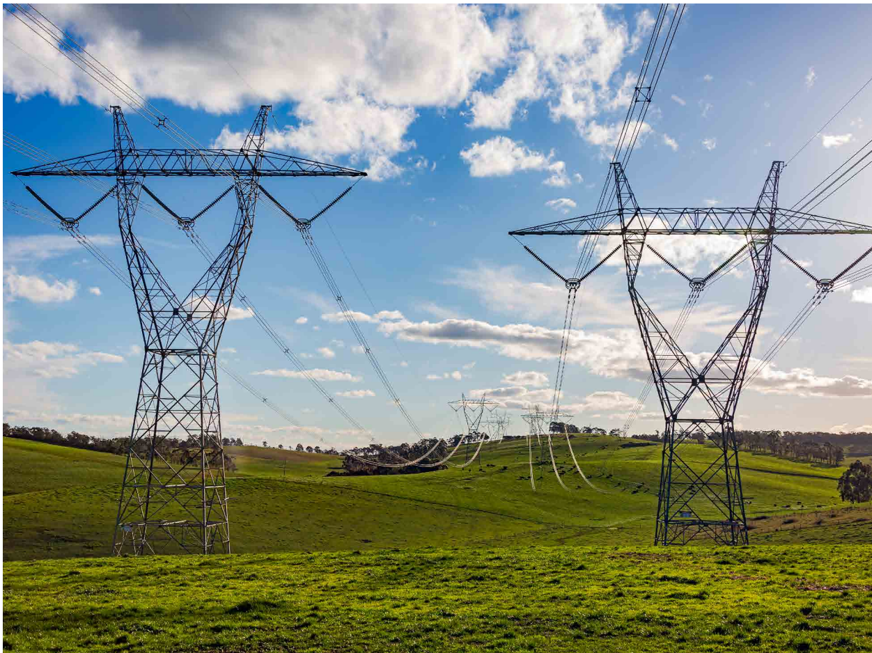
Power lines in rural Victoria.
