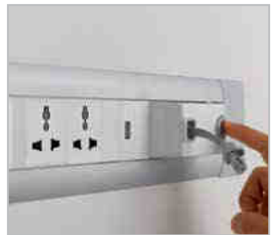
Flush mounting power & data module
