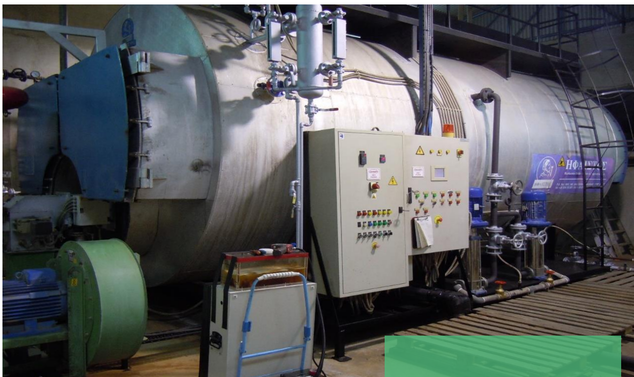
Figure 1: The use of hydrogen in the largest steam boiler in Cyprus.
