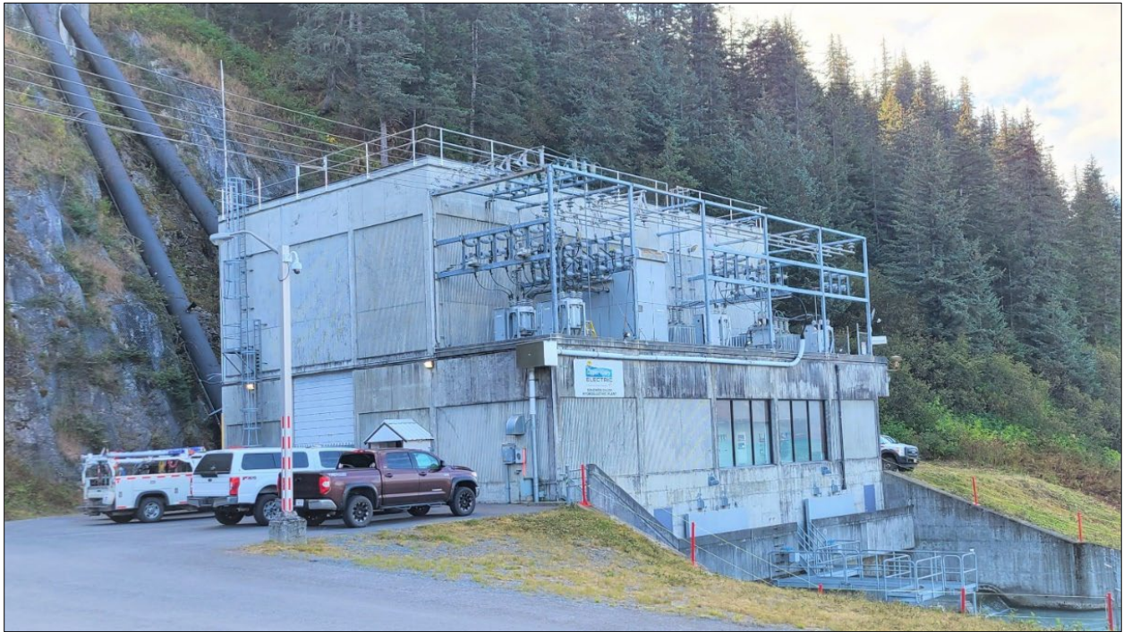
Photo 3-7 Solomon Gulch Project Powerhouse (Two Project Penstocks on Left)
