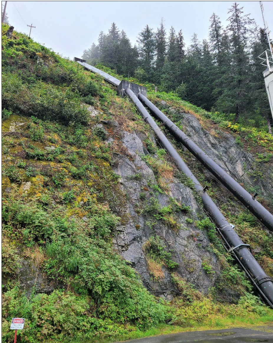
Photo 3-6 The Two Solomon Gulch Project Penstocks
