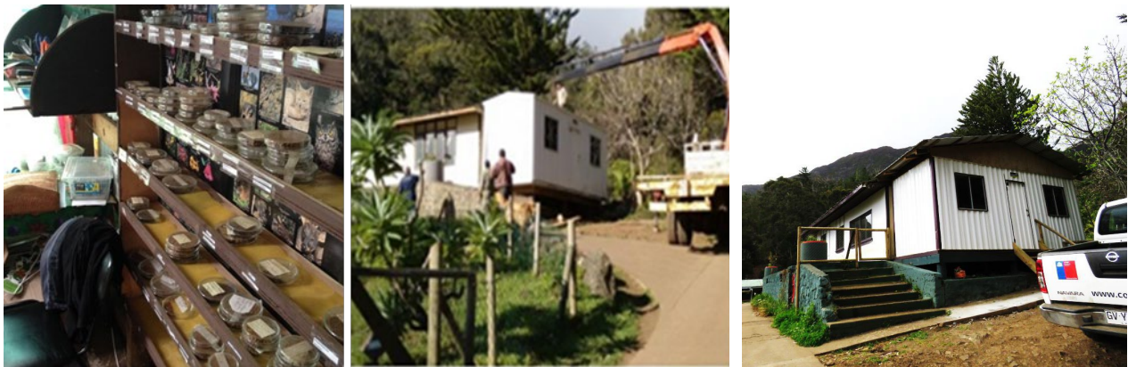
Figure 2. Installation of RCI seed bank. L-R: pre-project seeds stored on shelves in nursery; new seed bank structure installed; adjoining lab renovated.
