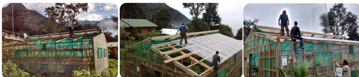
Figure 5. Essential repairs at the island's nursery, including a new roof and repairing damaged walls
