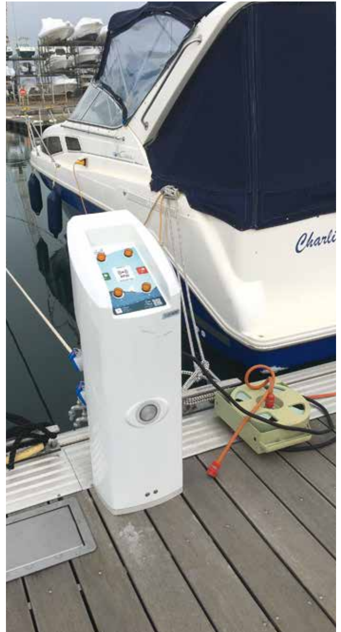
Example of personalised installation Sourcelec 278, Port Leucate, France
