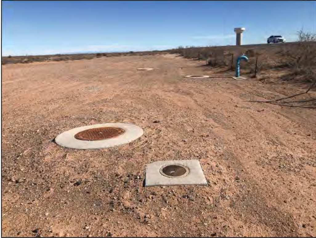
Photograph 3. Underground utilities installation located along the southern boundary of the proposed project area.
