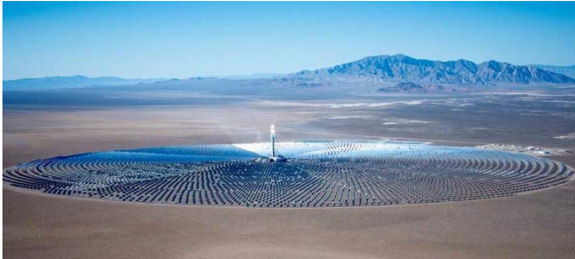
Fig. 2.1 – Typical Solar Energy Installation
