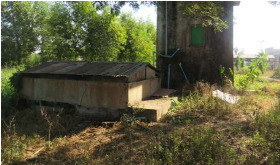
Figure – 39: Ground tank
