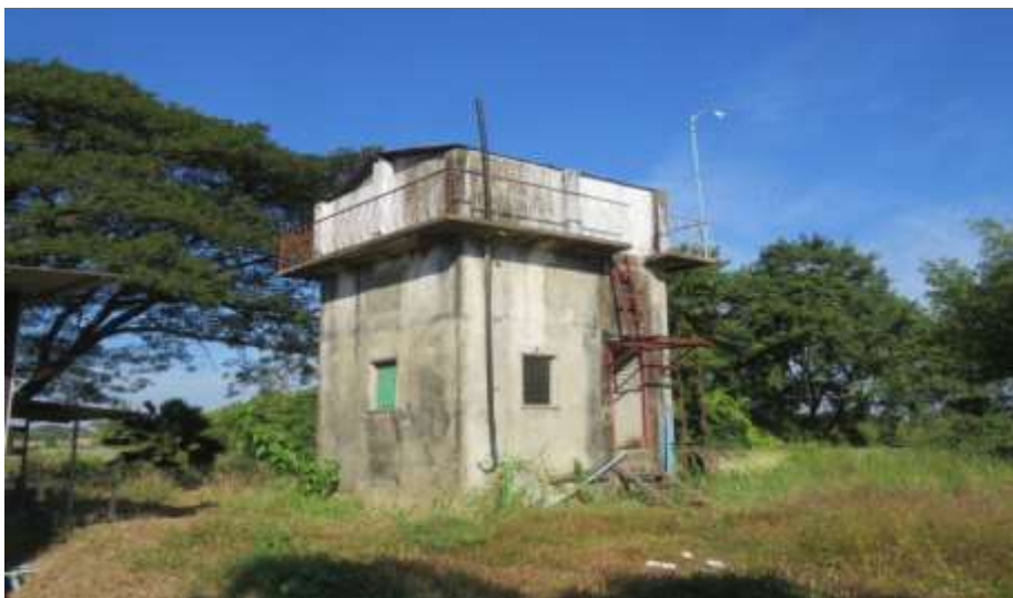
Figure – 40: Elevated tank
