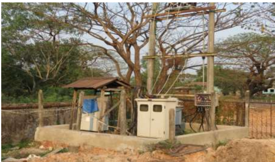
Figure – 56: Village transformer
