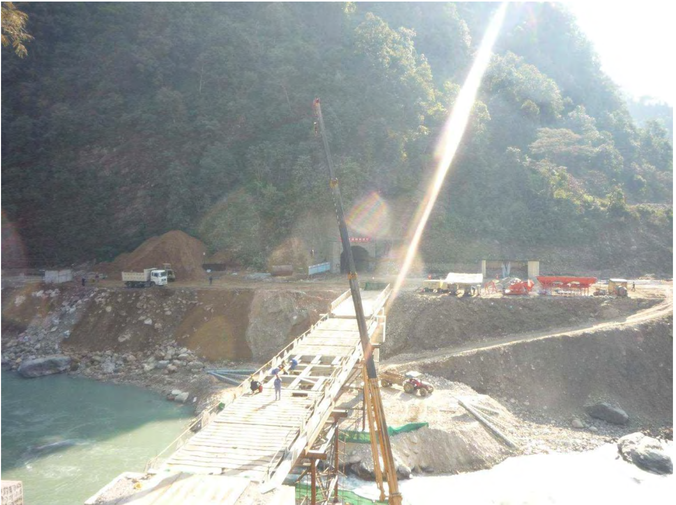
Figure 5: Construction of Upper Marsyangdi A near Khudi Substation site. Photo taken on Besisahar-Manang road which is inside the ACA.
