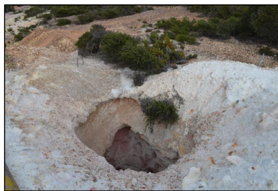
Plate 2: Unstable shafts in the Kundip mining area
