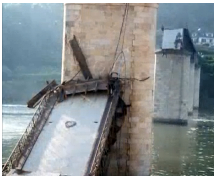
Figure 2. The bridge “Hintze Ribeiro” the day after it collapsed.
