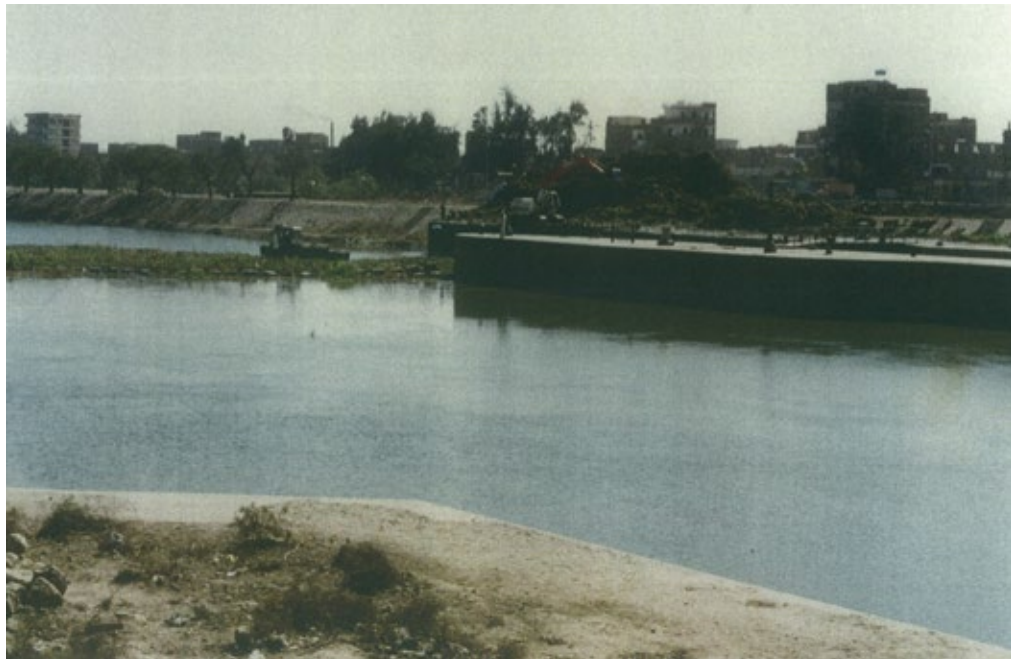
Figure 13. Removing water hyacinth upstream of a floating barrier by using a motorboat to move the weeds near the bank then removing them using hydraulic excavators
