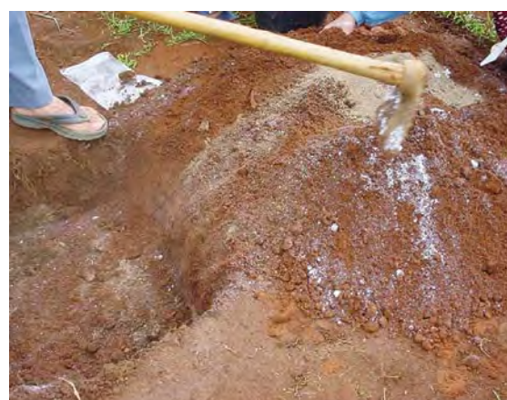
Figure 18. Procedure to follow when preparing the holes: 2 to 3 (top photograph); 4 to 6 (bottom photograph)
