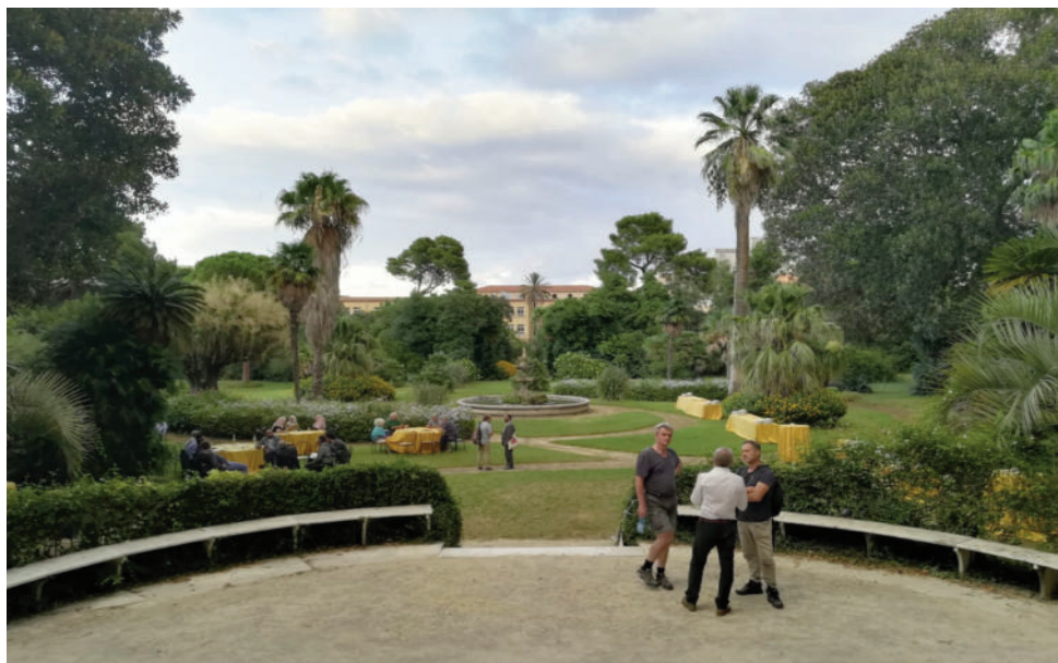
Villa Whitaker: overview of the garden during a break of the works.
