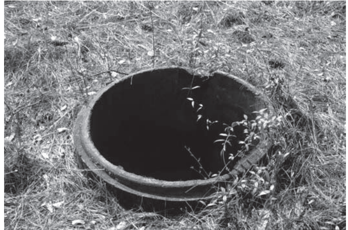
Figure 229 - Abandoned, uncovered water well
