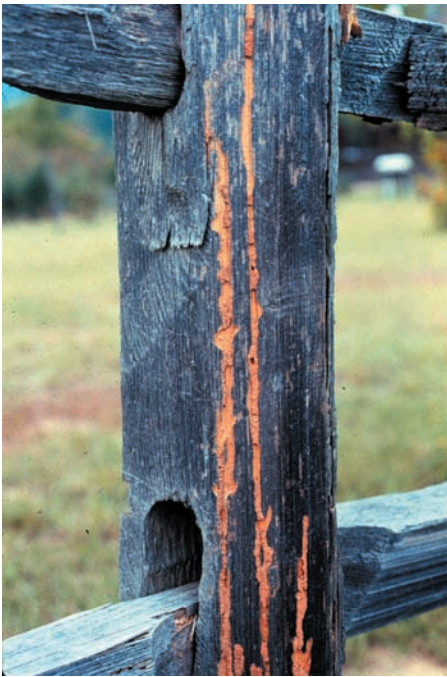
Figure 43 - Termite mud tubes on fence post
