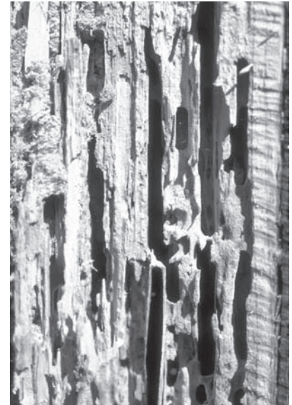
Figure 26B - Carpenter ant galleries
