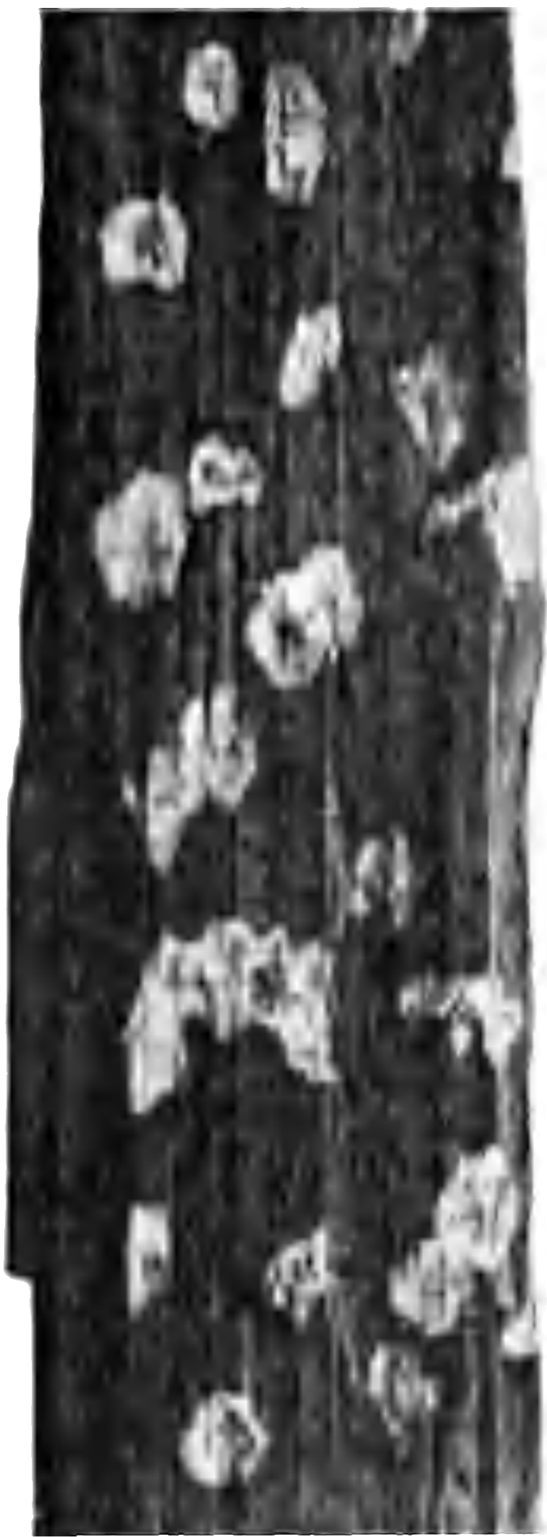
FIG. 23. — Pecky wood-rot; early stage in Douglas fir.
