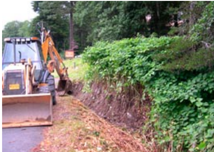
Figure 31. Roadside ditch maintenance can serve to spread Japanese knotweed.
