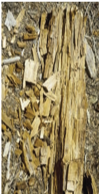
Figure 70. Brown cubical rot typical of Phaeolus schweinitzii . Photo: Joseph O'Brien, USDA Forest Service, Bugwood.org.
