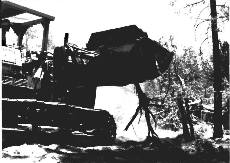
Figures 6 to 7. Removal of trees and stumps from six annosus root disease centers on the San Bernardino National Forest. Upper, pushing over one of the pines; lower, piling uprooted materials. (Photos courtesy USDA-Forest Service).
