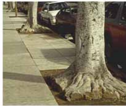
Trees roots have been cut to avoid sidewalk damage. This is a recordable damage.
