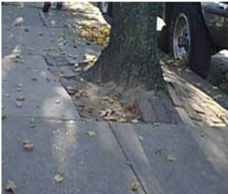
Figure 7.70: Sidewalk conflicts with roots.
