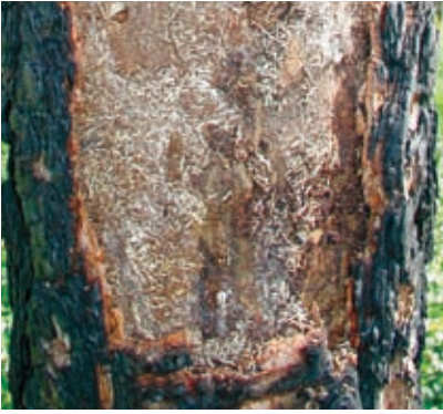
Figure 486. White, splinter-like boring frass produced by roundheaded wood borers when feeding. Photo: Sheryl Costello, USDA Forest Service.
