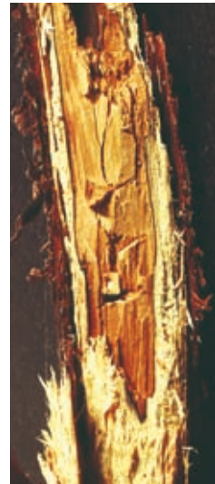
Figure 31. Dead, decaying stem with white rot in the outer wood and brown rot in the inner wood caused by two different fungi. The white rot is stringy-fibrous; the brown rot breaks easily across the grain, has no fibrous strength, and is crumbly when dry. Photo: Jim Worrall, USDA Forest Service.
