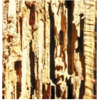
Figure 458. Carpenter ant damage. Photo: Edward R. Werner, USDA Forest Service, Bugwood.org.
