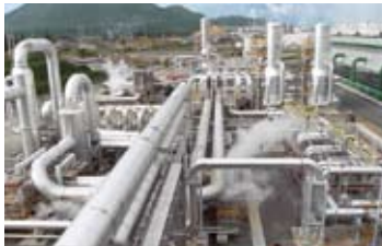
Geothermal power generation plant
