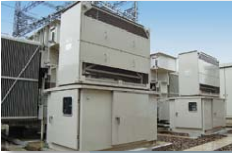
Power Receiving and Distribution Substation Equipment for Railway Companies
