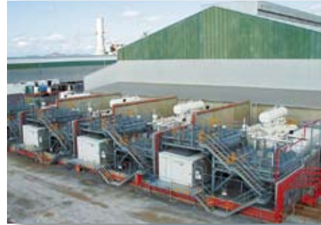
Substation Equipment for Aluminum Refinery We have supplied substation equipment including high-capacity rectifiers (equipment that convert alternating current to direct current) as primary power supply equipment for aluminum refineries in the Middle East.
