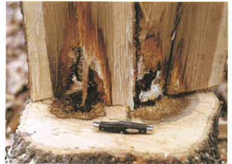
Decay caused by shoestring root rot fungus.
