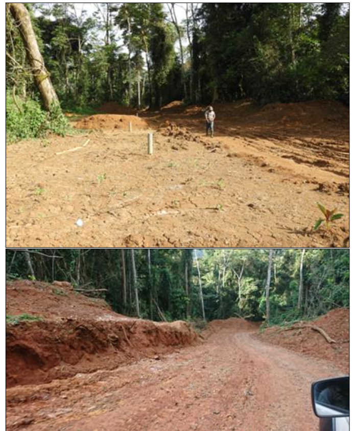
Fig. 3. Areas of forest cleared in 2019, to create access routes and geological survey stations.
